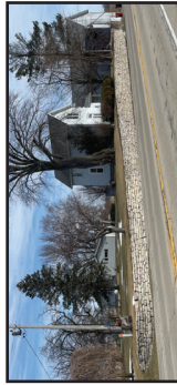
10 Available off-road trail space is limited due to a retaining wall adjacent to HWY 60.
