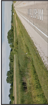
7 Drainage swale/culvert adjacent to R.O.W. may limit grading or require boardwalk.
