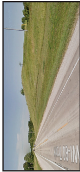
⑥ Steep side slopes in R.O.W.
