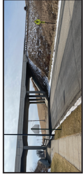
① HWY 60 overpass above S Hustis St creates narrow R.O.W. conditions for trail crossing.
